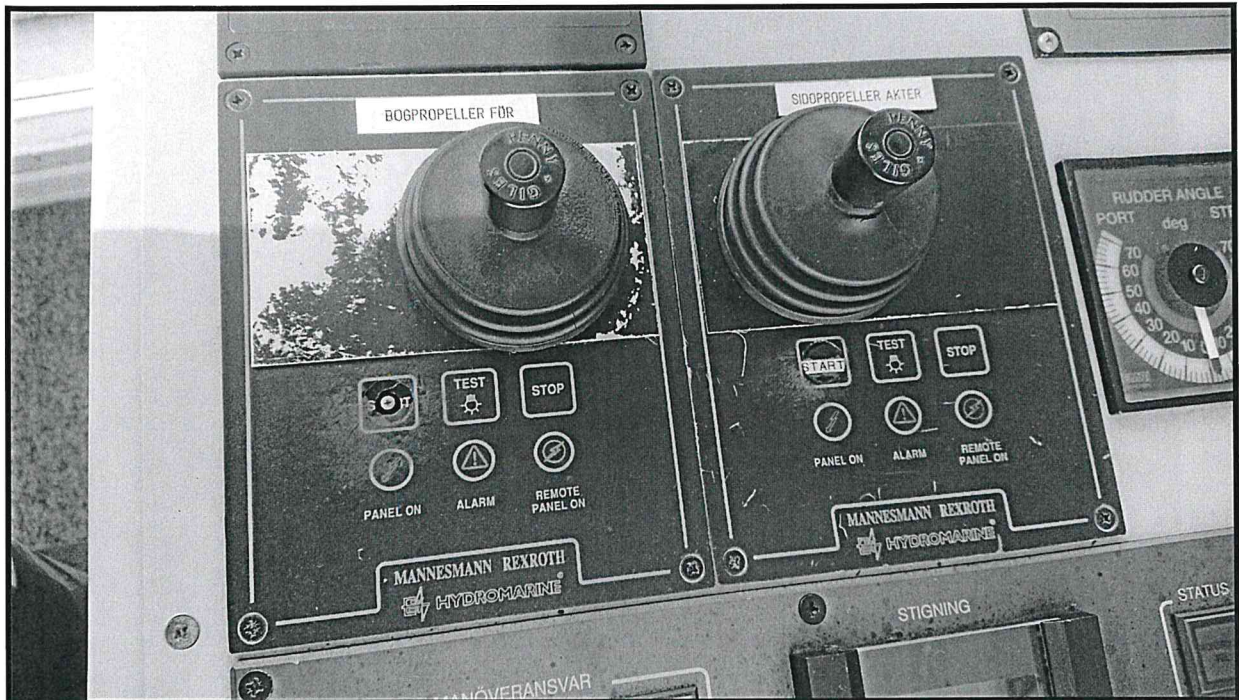
Picture 1. The existing transversal thruster controls at centre console.
