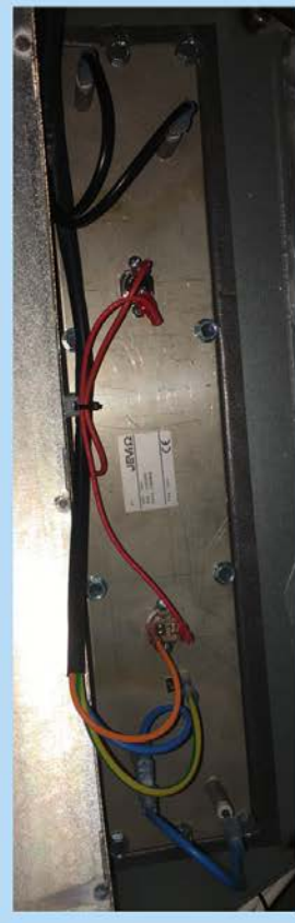
Electric heater foto
